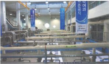
Yeongdeungpo Drinking Water Treatment Plant in Seoul Client ----- Seoul City Capacity ----- 25,000m 3 /day
