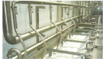
Drinking Water Treatment Plant in Nongfu, China Client ----- Nongfu Spring co., China Capacity ----- 6,720m 3 /day
