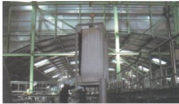
Guri I 3 System Sewage Treatment Plant Client ----- Guri City Capacity ----- 26,250m 3 /day
