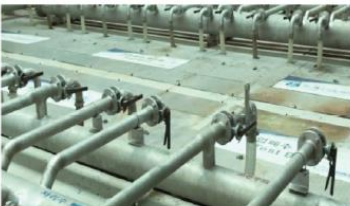
Gumi K Factory Wastewater Treatment Plant Client ----- K company Capacity ----- 10,000m 3 /day
